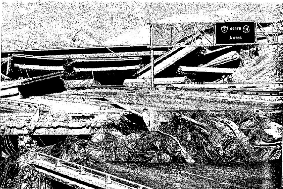
FIGURE 8.23 Damage to Interstate 5 caused by the January 17, 1994, Northridge earthquake. (Photo by Tom McHugh/Photo Researchers, Inc.)
